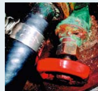
Many used boats have gate valves. This one is terminally corroded
