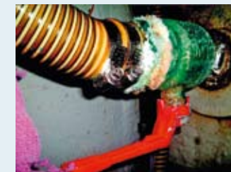
Most modern boats have gate valves. This one needs replacing
